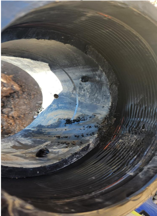
Failed coupler due to poor alignment
