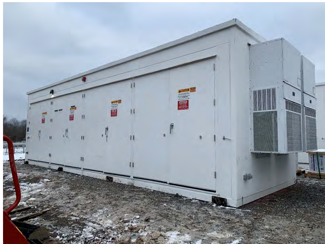
5 MW Direct Current (DC) BESS: New York
